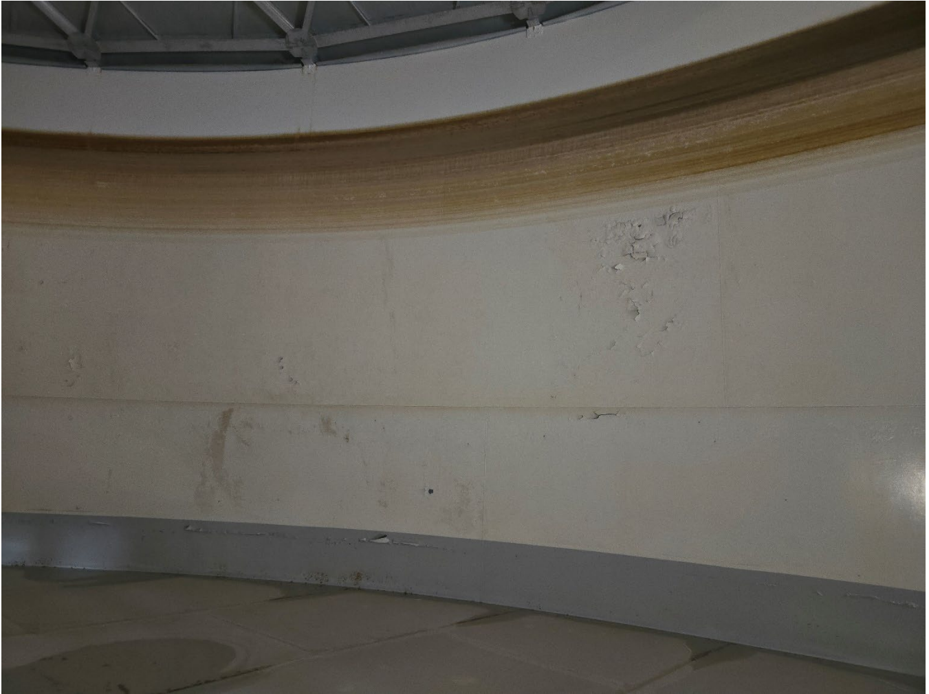
Interior coating delamination on tank sidewall
