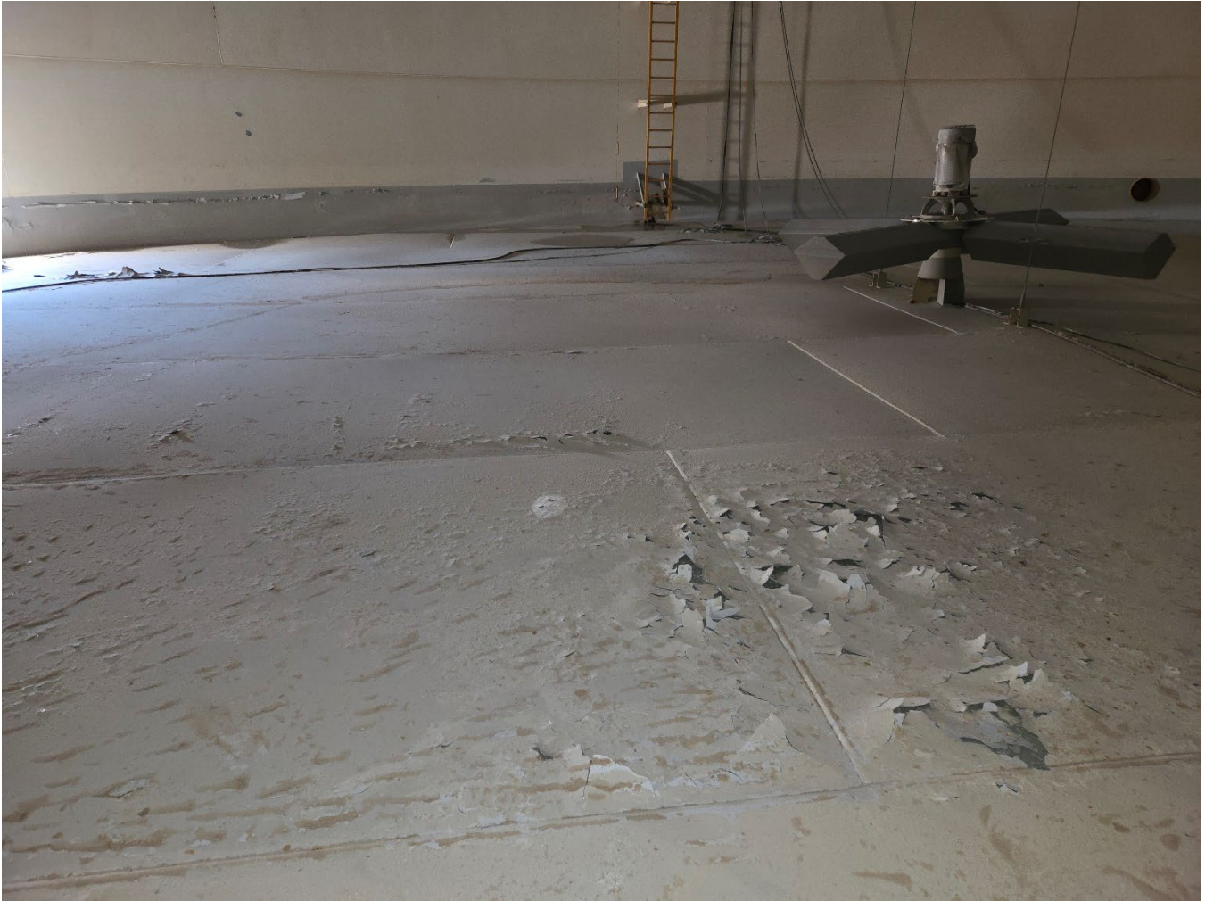
Tank floor showing significant interior coating delamination
