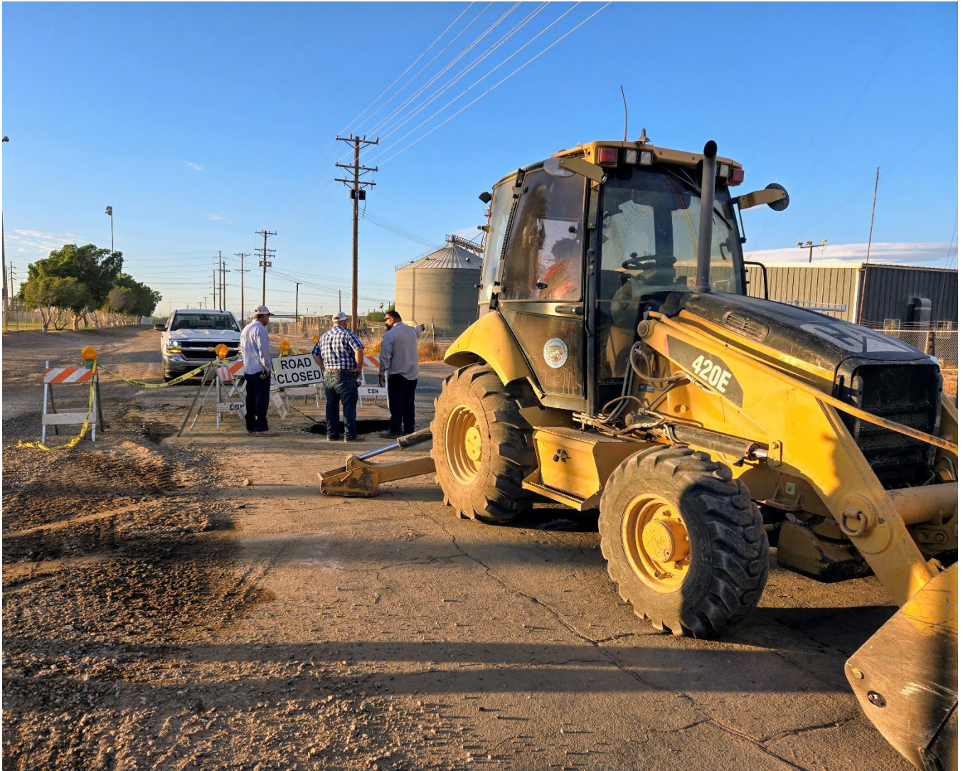
Public Works staff responding to collapsed manhole.
