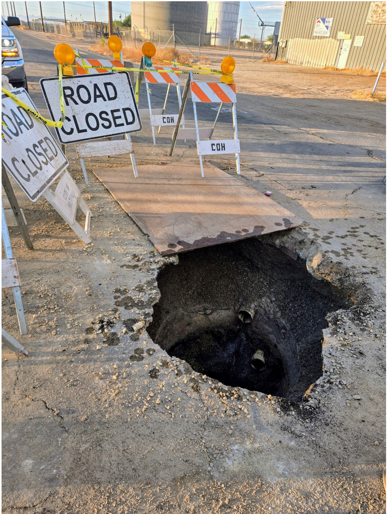
Close up of view collapsed manhole.
