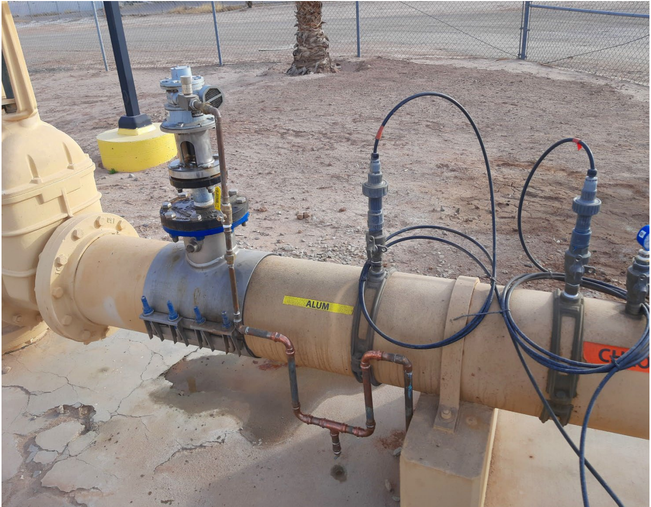
Water plant staff completed repair work and re-installation of raw water chemical pneumatic flash mixer and placed back into service.
