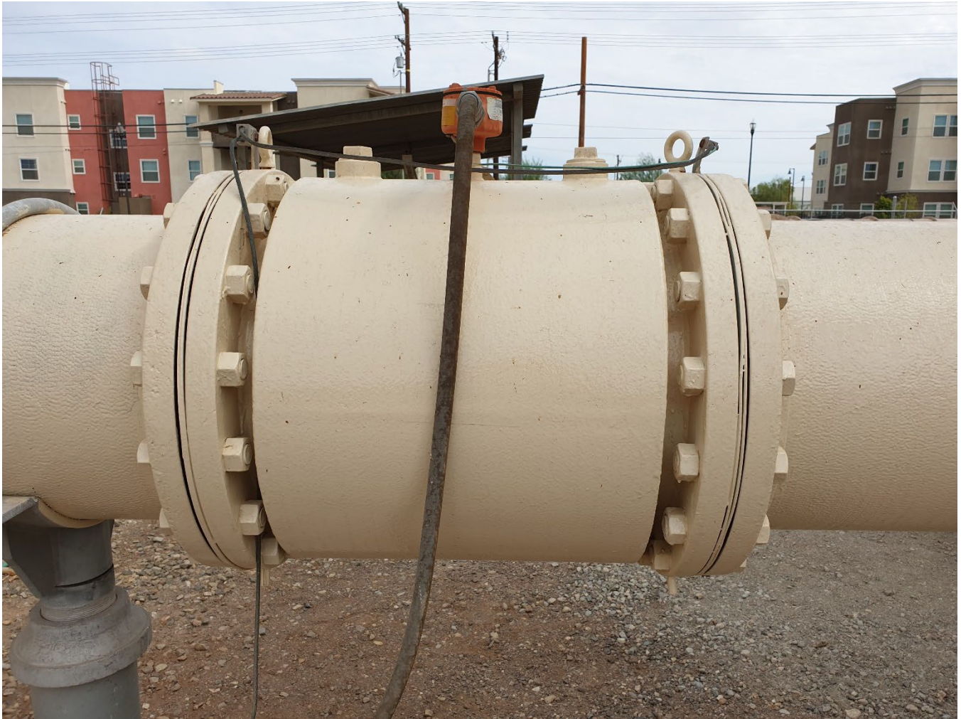
2.4 MG Tank TigerMag flowmeter in service while repairs are made to main distribution flow meter.
